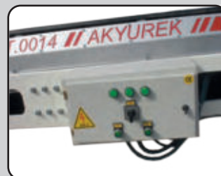
On Board Power Panel
